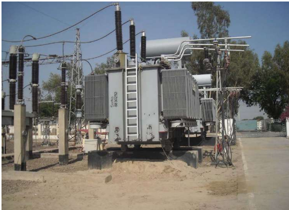
132 KV Grid Station Kacha Khu
