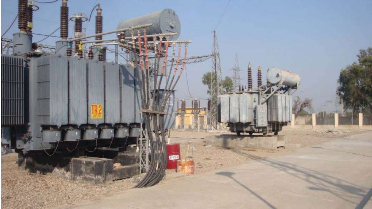
132 KV Grid Station Kehror Pakka
